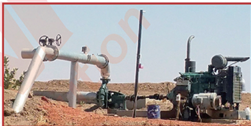
Hook up for pump with diesel engine
