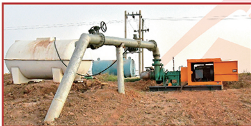
Hook up for pump with motor
